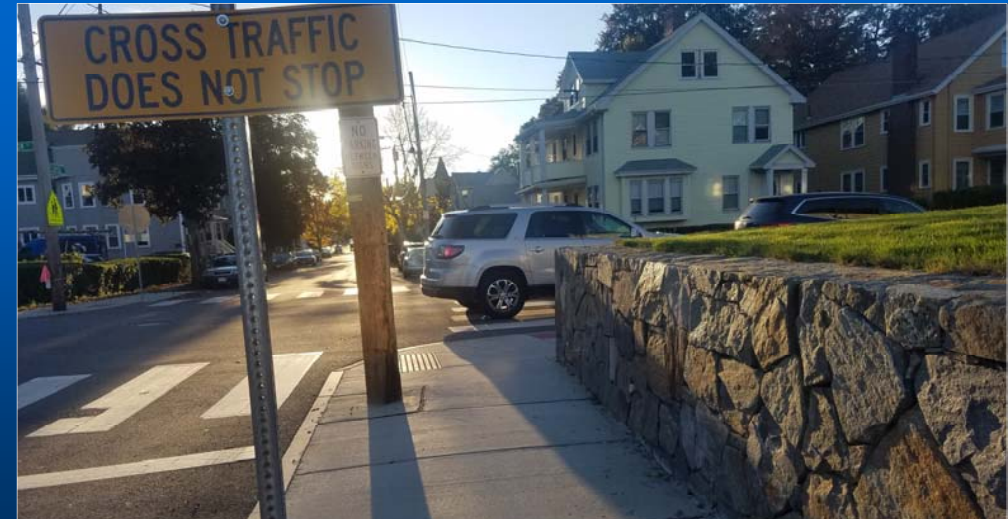
Stone wall causes poor sightline for westbound approach
