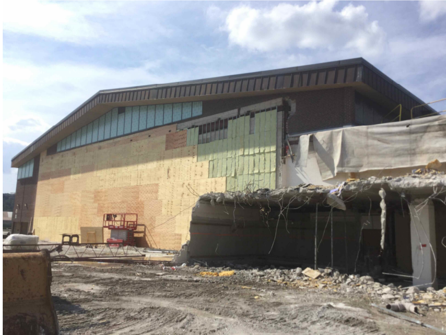
Photo 2 – Demolition Progress of Locker-Room Structure / Framing, Insulation and Plywood of Field House Exterior Wall for Weather Protection.
