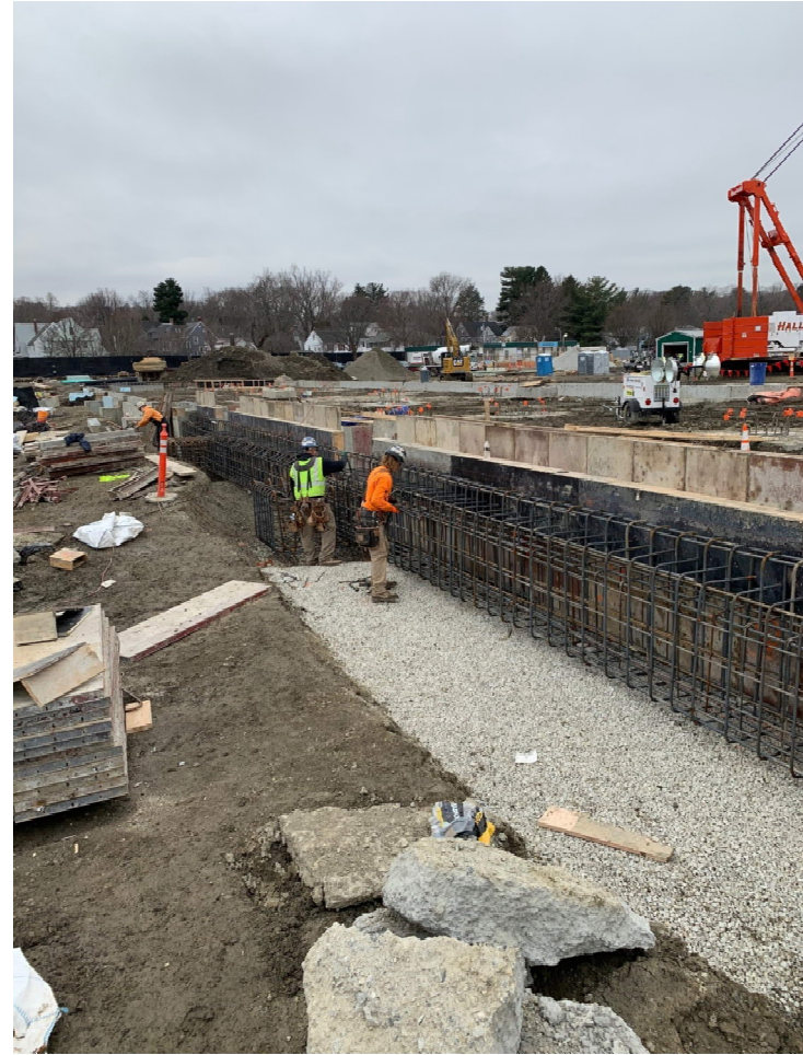
Photo 2 – Forming J Line Grade Beam for Final Concrete Placement of Foundations for Phase 1.
