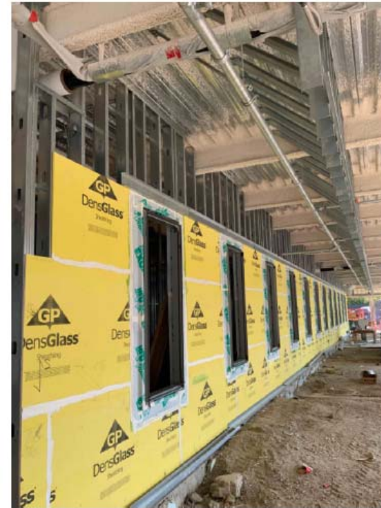
Photo 10 – Exterior Sheathing and Window Frames on Level 1 of Area A, West Elevation
