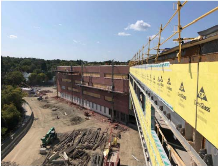
Photo 9 – Installation of Bick Façade at Area A and Exterior Sheathing at Area C (Southeast Elevation)
