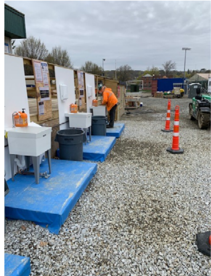
Photo 13 – Trades Using Permanent Hand Wash Stations.
