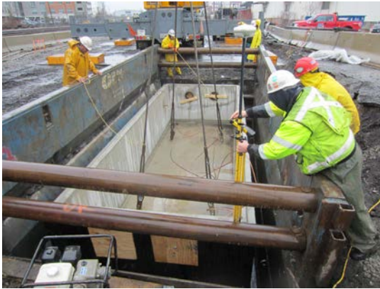
Construction crew works on installation of the Transmission line pipeline in April 2016.
