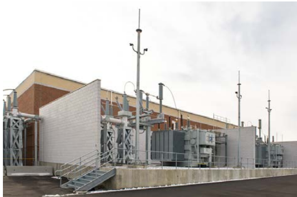
Back side of the completed Blair Pond Substation, showing the new transformers, in late 2016.
