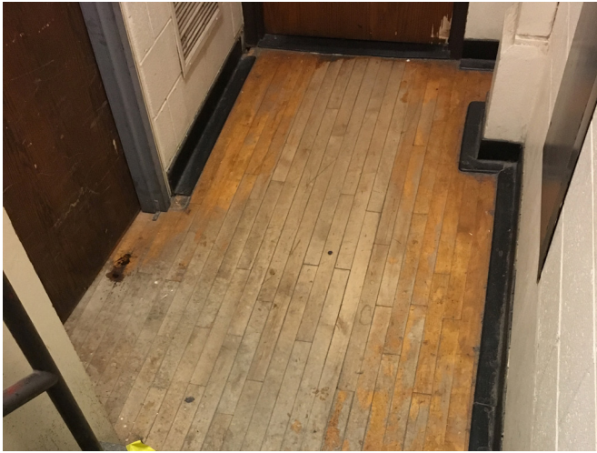
Worn wood flooring at wood shop and orchestra room
