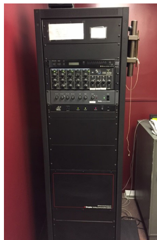
Intercom System in Office Area
