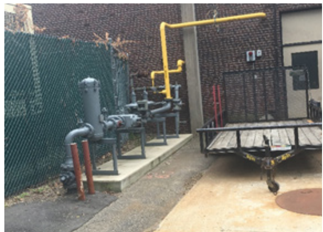
Figure 6: Gas meter along the north of the School
