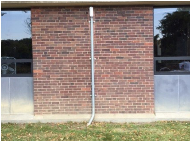
TELCO Entry Point
