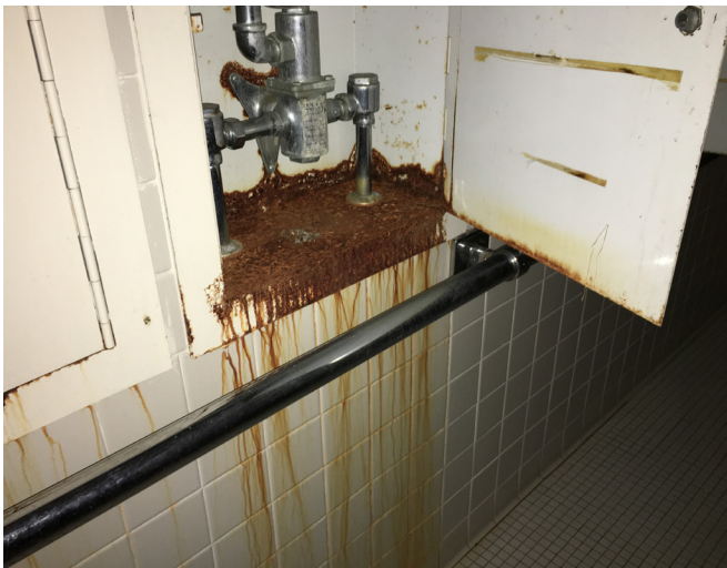
Corroded piping and wall
