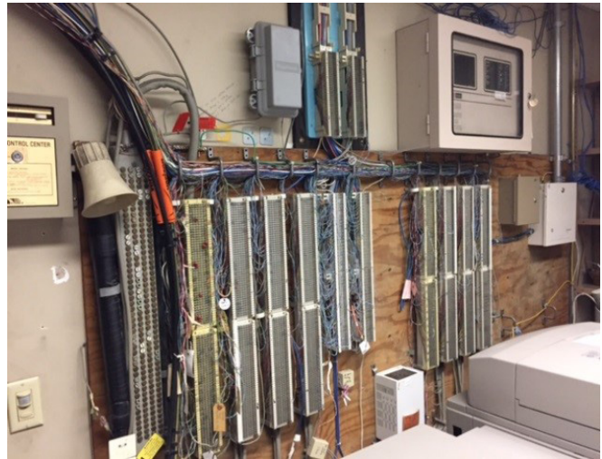
Typical IDF Wall Mounted Cabinet
