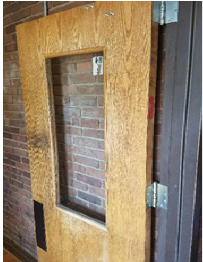
Figure 3: Rated Stair Door with no Latch and Non-rated Glazing
