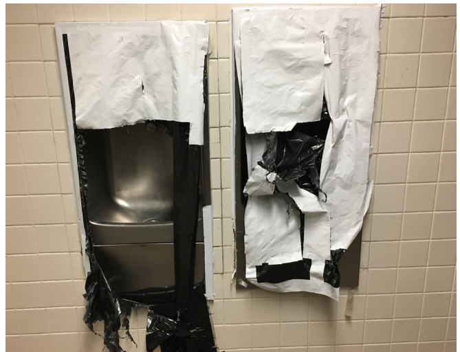
Water faucets inoperable
