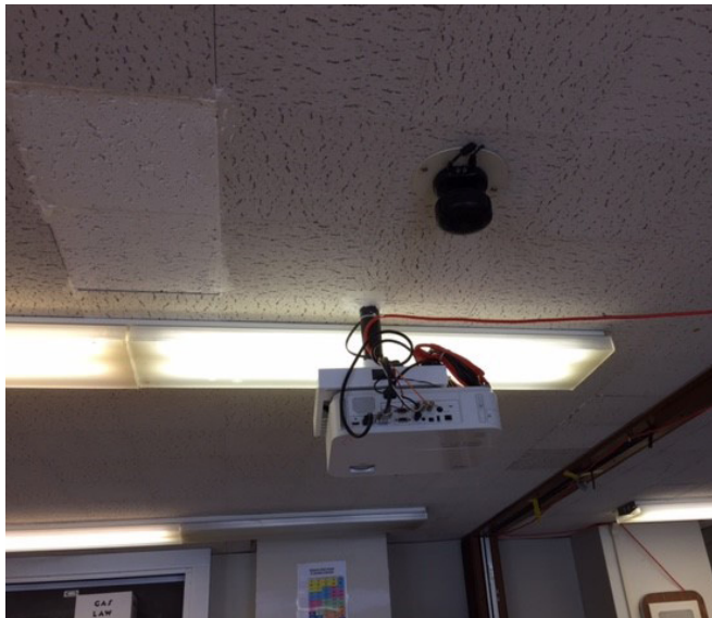
Typical Classroom Projector Setup
