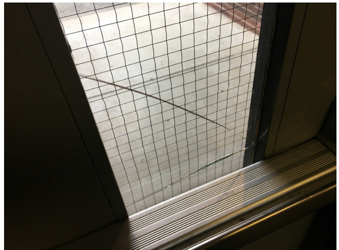
Broken glass in window panel
