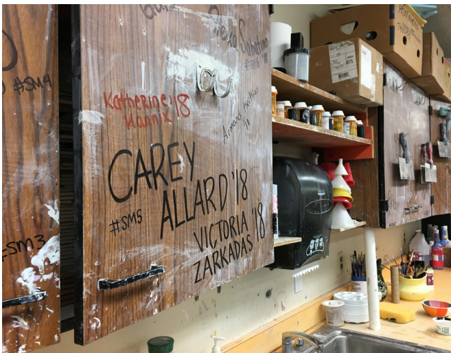
Cabinet and shelves in deteriorated condition
