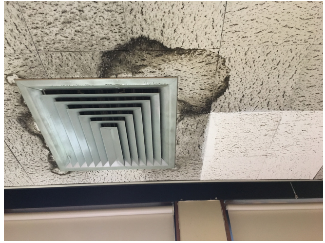
Water damage at ceiling diffuser
