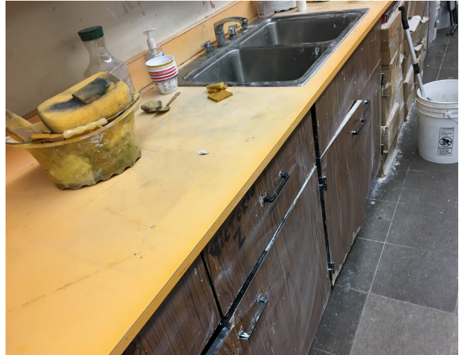
Cabinet and countertop in deteriorated condition
