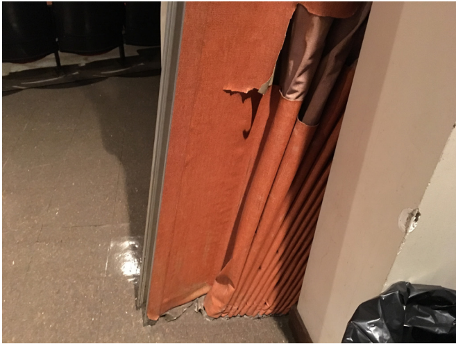
Damaged coil Wall partitions in auditorium
