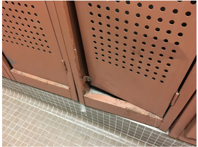
Deformed locker door
