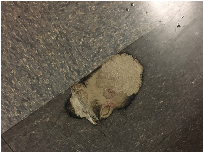
Flooring worn out at door locations
