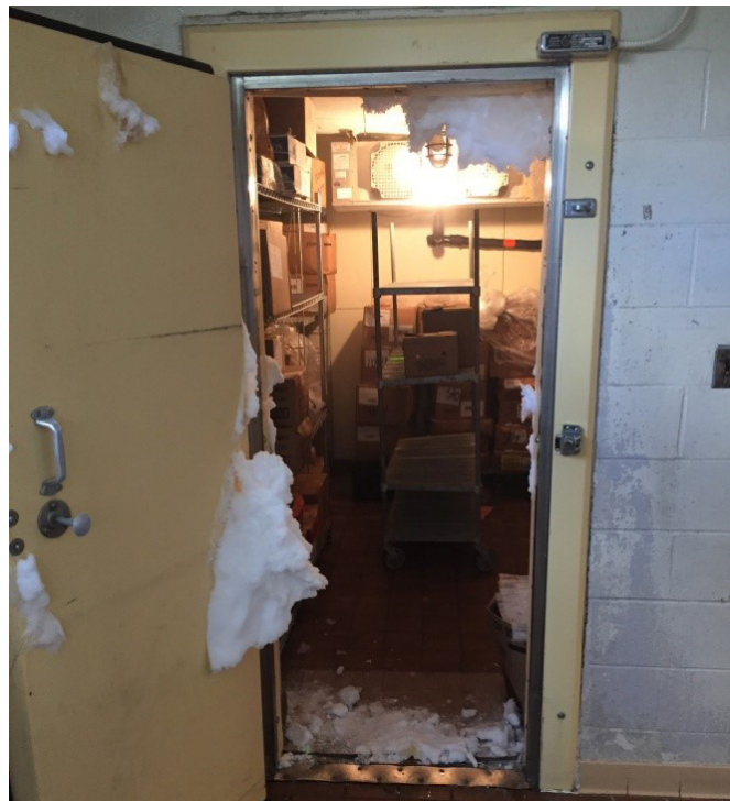
The walk-in refrigerated rooms are old and constructed from masonry with a stucco rough texture finish on the walls and ceiling. The picture above shows mold spores growing on the surface of the ceiling. The picture above shows ice build-up around the door frame which is indicative of poor room insulation and broken or missing door seals. A new walk-in will provide additional storage capacity and Energy Star rated refrigeration systems that will save energy. It'll provide insulated walls and door panels to that meet the requirements of the National Sanitation Foundations. The panel surface finishes will meet the board of health requirements for cleaning. Doors will be equipped with a view port window for safety.
