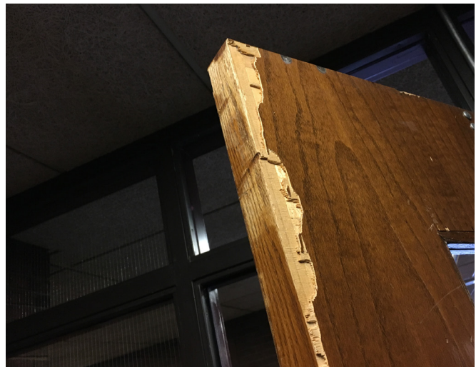
Cracked and damaged wood doors
