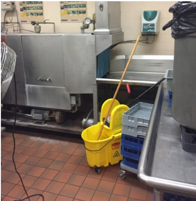
The dish machine pictured is at least 10 years old. A new Energy Star rated unit will save a significant amount of water use, sewer cost and electrical demand.
