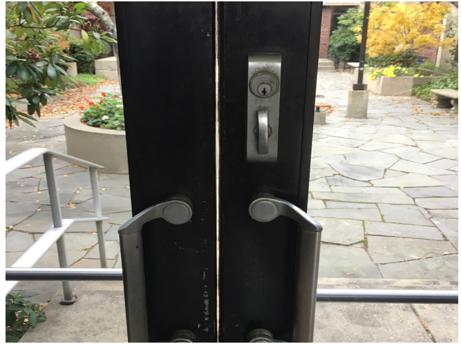
No thermal barrier between doors
