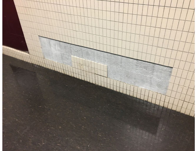
Tiles falling off the wall
