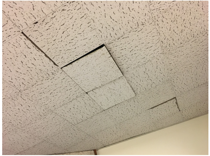
Misaligned ceiling tiles
