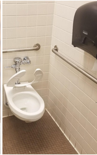
Figure 12: Toilet Paper Dispenser above Grab Bar
