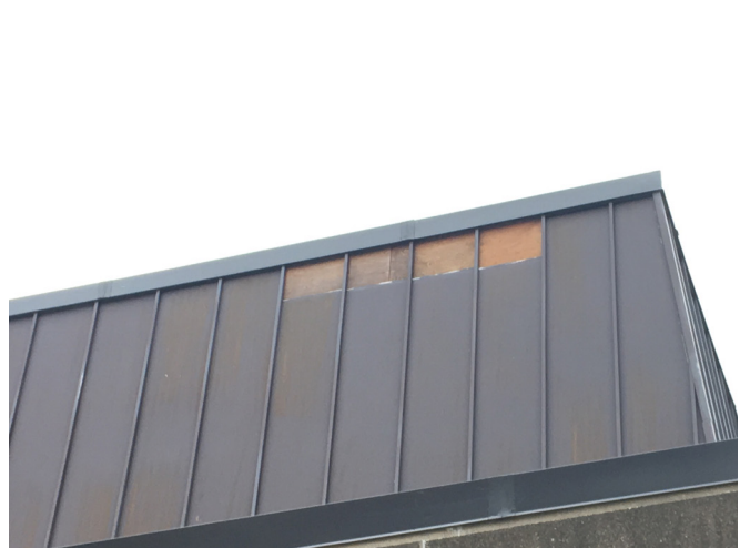
Exposed exterior wood substrate at theatre
