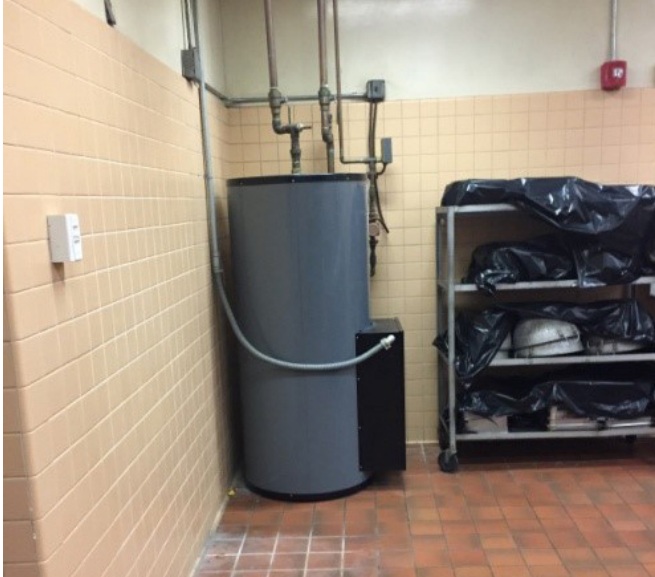
The hot water heater should be located in a dedicated room away from all food production operations.
