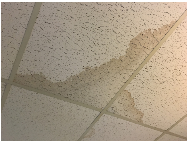
Water damage at ceilings
