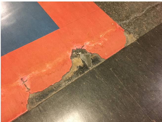
Severe cracking of floor tile
