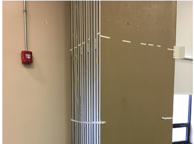
Damaged coil Wall partitions in cafeteria
