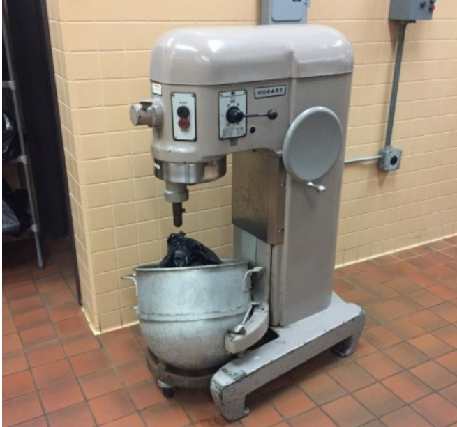
This mixer should be replaced with the new unit that provides protective safety guards and stainless steel mixing bowls. The peeling paint on the body of the unit is not allowed by the board of health.
