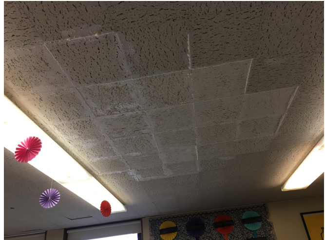
Ceiling modification due to water damage
