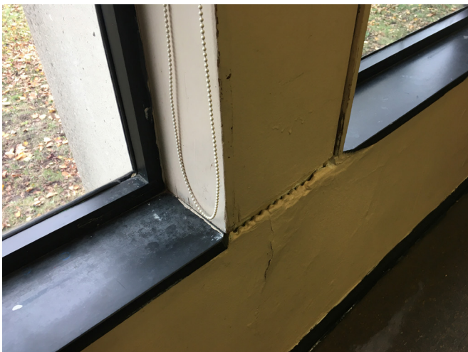
Cracks in wall finish
