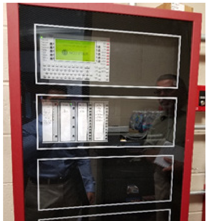
Figure 4: Fire Alarm Control Panel
