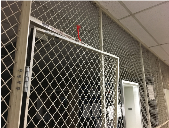
Damaged locker room door
