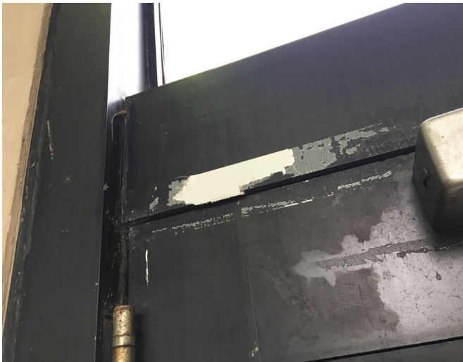
Paint damage at the door
