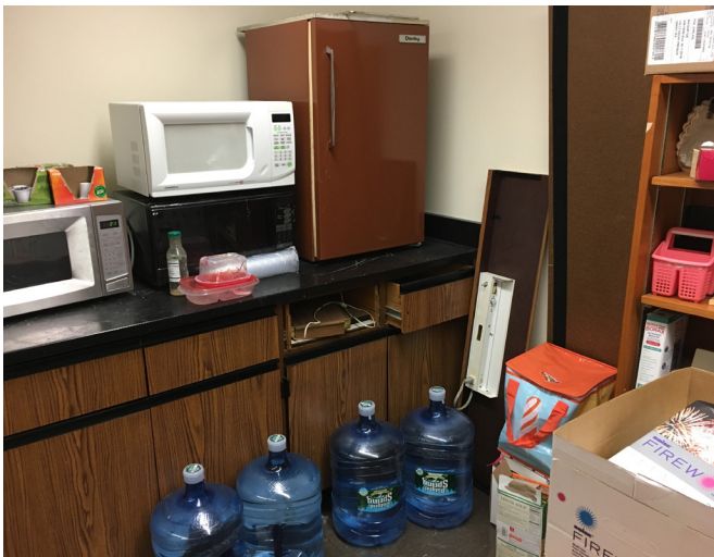
Damaged cabinet drawers
