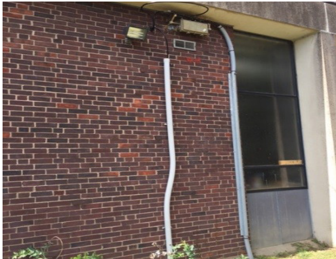
Fiber Optic Entry Point
