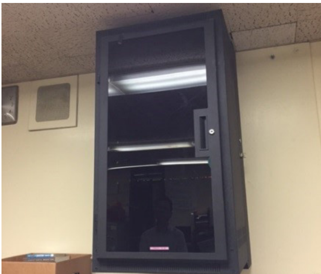
Typical IDF Wall Mounted Cabinet
