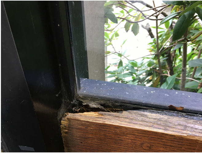
Water damage at window
