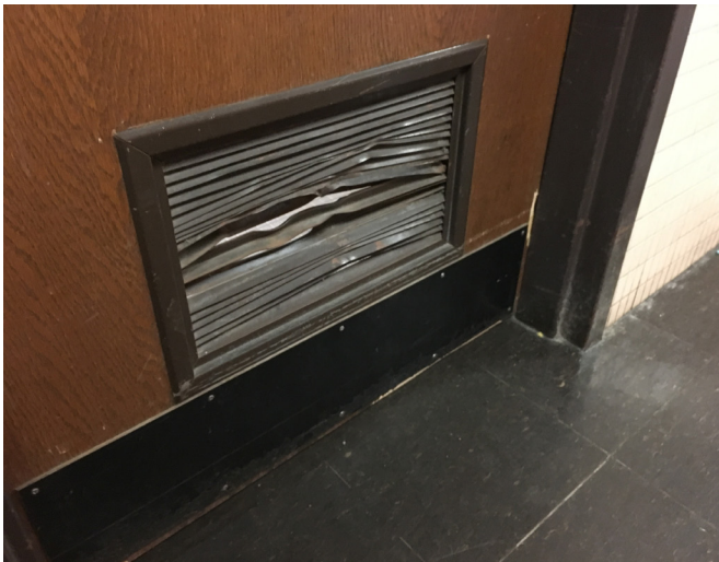
Damaged door louver
