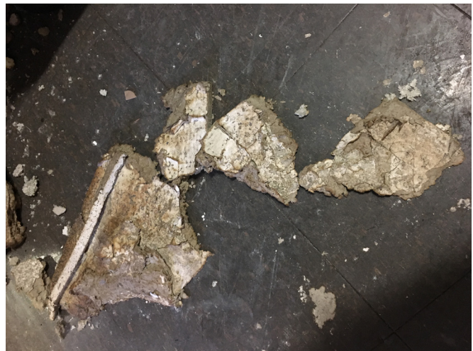
Falling ceiling tiles due to water damage
