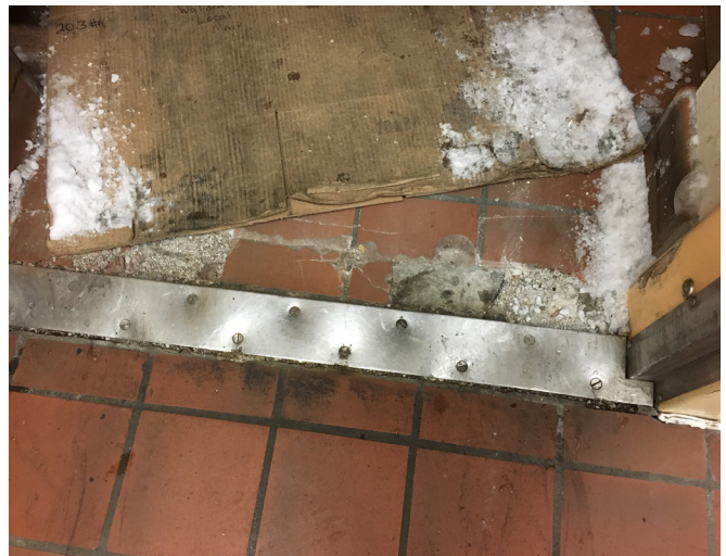
Tile damage at kitchen freezer
