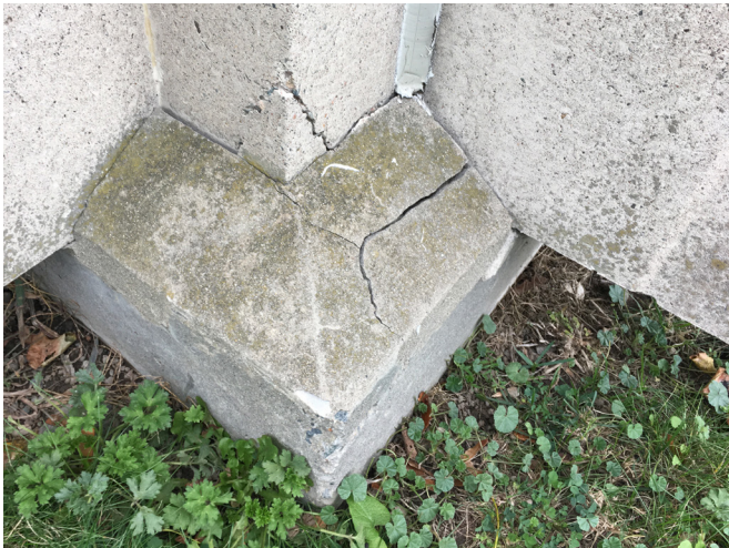
Deterioration throughout exterior concrete
