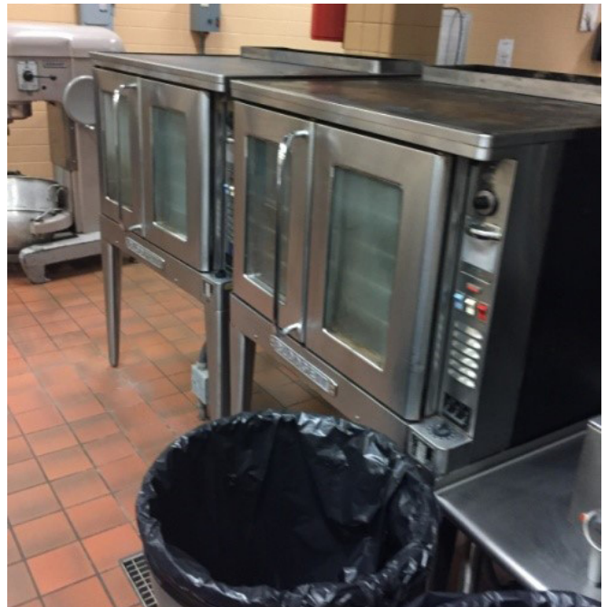
Shown here are two single convection ovens which are nearing the end of the life cycle (ten years). New gas fueled units are Energy Star rated which qualifies them for a rebate from the gas company.
