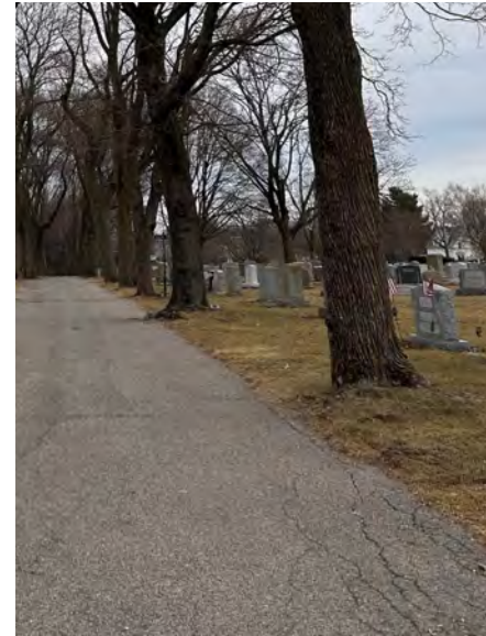
Edge cracking on South Avenue
