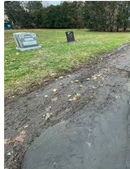
Rutting on Norton Circle
