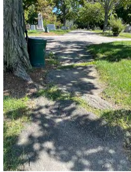
Tree root impacting a narrow walkway on Lilac Circle
