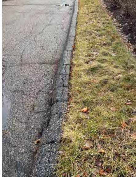
Cracking of bituminous curb at the heart bed
