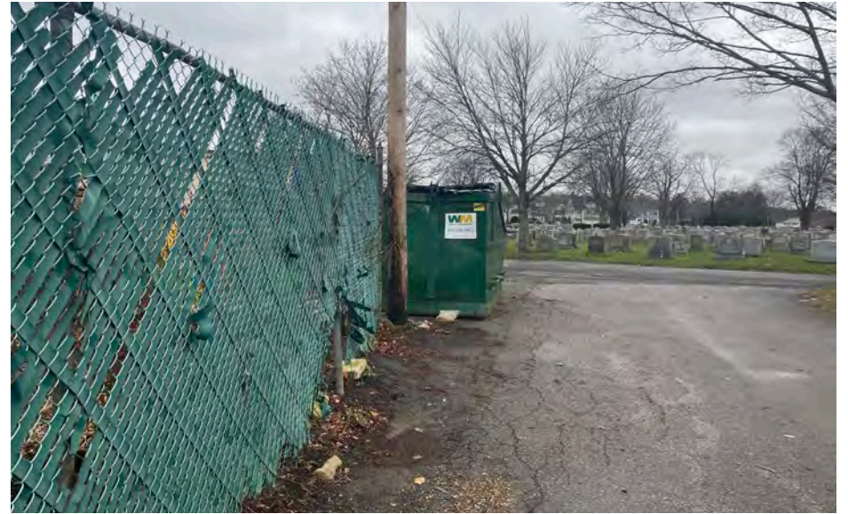
Condition of fence fabric and privacy slats
