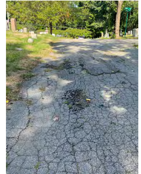
Alligator cracking on Orchid Avenue
