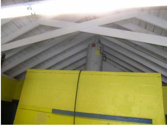
Hot Water Heater
