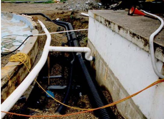
Pool Return Lines Installed in 1995
