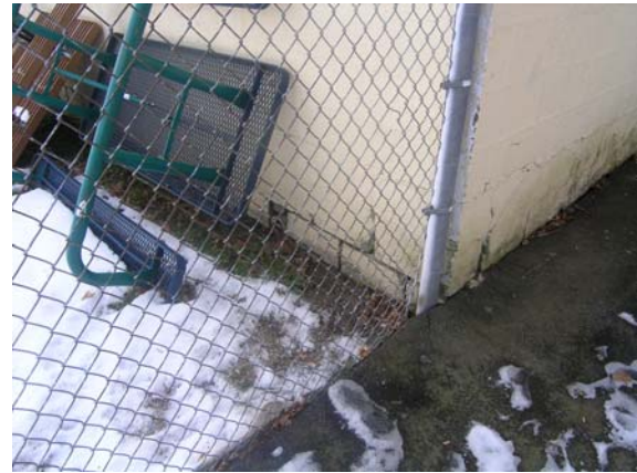
Open Masonry Joints at northwest corner.
