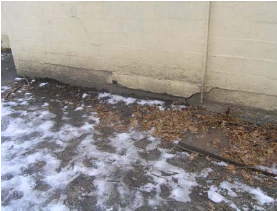
Cracking at West Elevation
