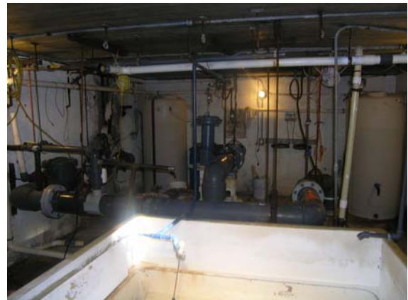
View of space over filter.
