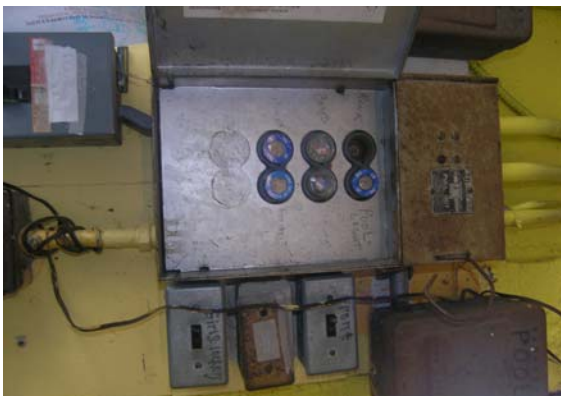
Sub-panels in lobby
