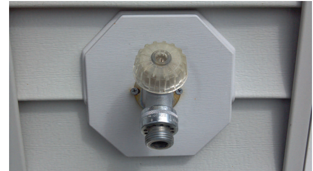
Vacuum Breaker installed on hose bib connection
